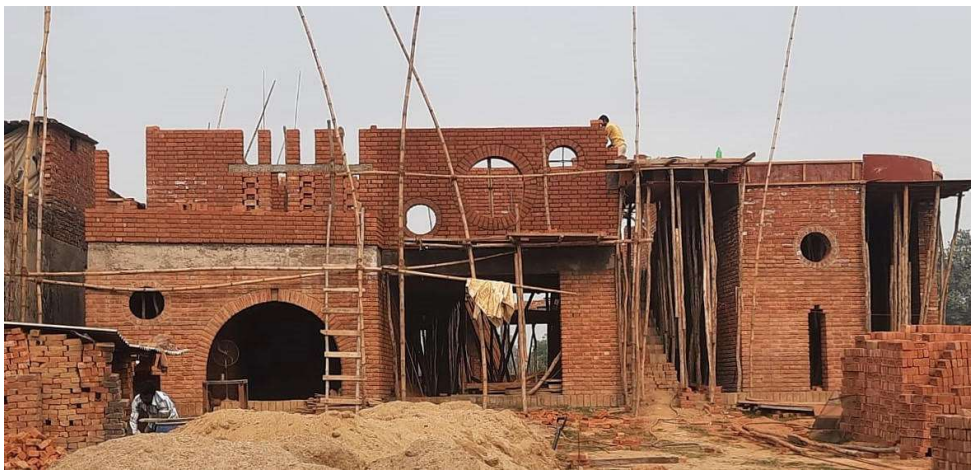
And here's the new front view. The second floor is now complete except for the roof which will be poured in a few days. The tall space to the right of the 3-round-window wall will be the stairwell.
